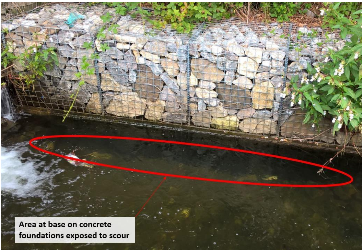
Figure 4 – Section 2: Gabion foundations exposed to scour
